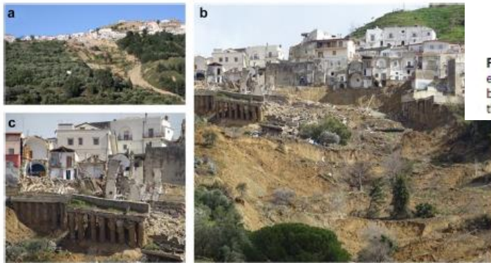
Fig. 2 Photos (taken by the authors during the field surveys) of the Pomarico clay rotational-planar slides (sensu Hungr et al. 2014). a The January 29th, 2019 event; b landslide crown and the collapsed buildings and road located along Corso Vittorio Emanuele II; c detail of the bulkhead breakdown
